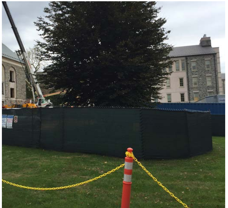
Tree protection zones minimize the effects of construction damage when enforced.
