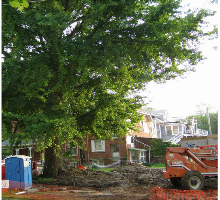
Workers ignored this tree protection zone. Heavy equipment and materials stored on the root system will have significant consequences.
